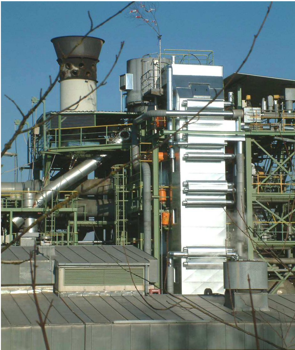
Combustion chamber with steam boiler
